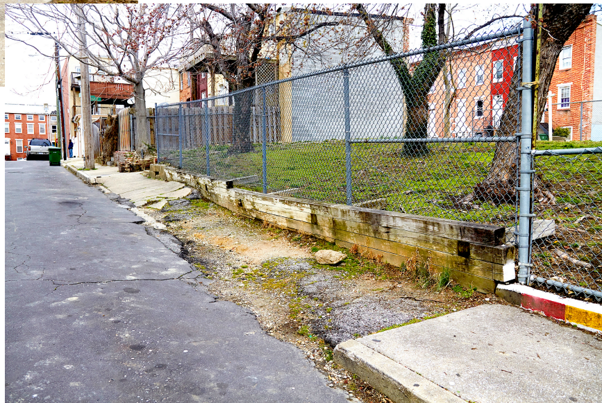
Blighted sidewalk in need of repair
